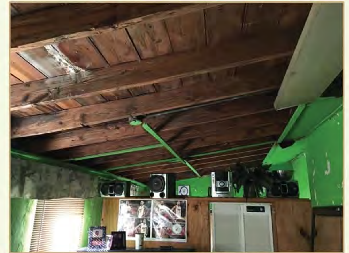
Interior damage from Hurricane
